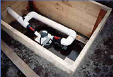
Stream Engine Installation: 8 meter (25 foot) head, 450 Watt output
