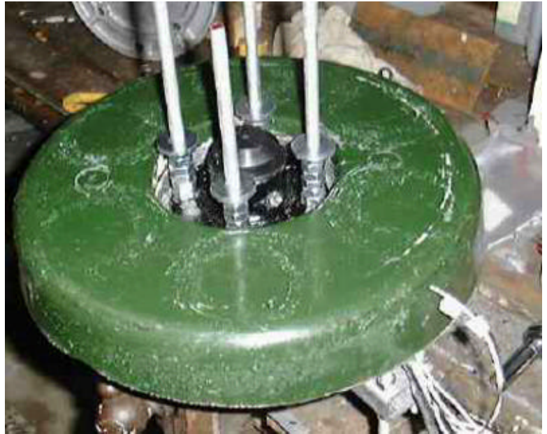
Fitting the stator
